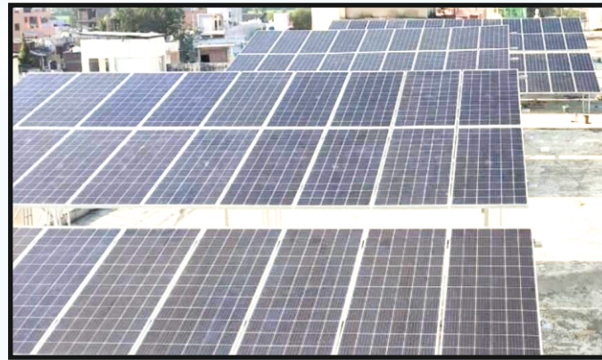
SATYAM MOTOR MARUTI SUZUKI, BHOPAL PROJECT CAPACITY-60KW, COMMISSIONING DATE-JUL 2020
