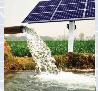
Solar Water Pump
